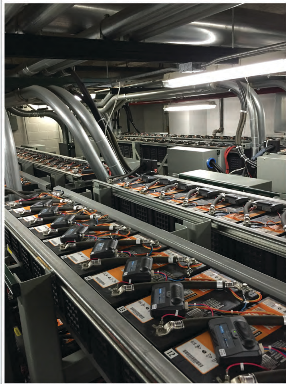
Dedicated Battery Room for UPS Systems.
