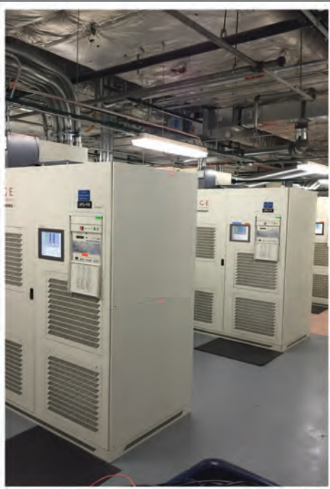
UPS System 6, 7 and 8.
